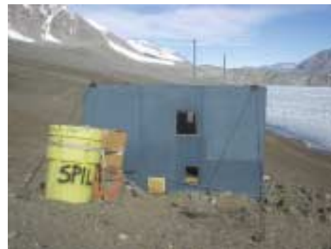
Diesel Gen Shed at Lake Bonney
