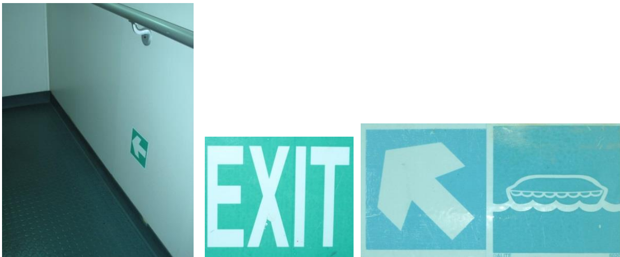
Figure 3: Egress Arrow, EXIT Sign (to weather deck), and Life Boat Arrow
